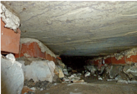
View north under the north aisle of the nave, showing the underside of stone slabs supported on brick and stone sleeper walls. The slabs form the substrate of the 'medieval' tiled pavement above
